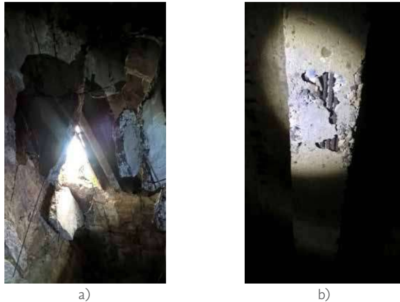
Figure 5. a). Slab collapse and b). Areas without concrete cover and with visible concrete segregation in beams of the RC structure
