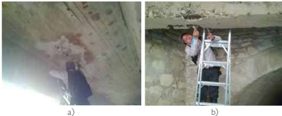
Figure 14. a). Measurement of deterioration (segregations) in slab and b). Measurement of beam's segregations with digital vernier "Mitutoyo" and transparent millimetric ruler
