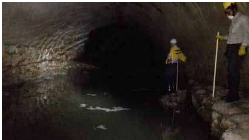
Figure 2. Black water flowing through the "San Roque Underground culverts-arch"
