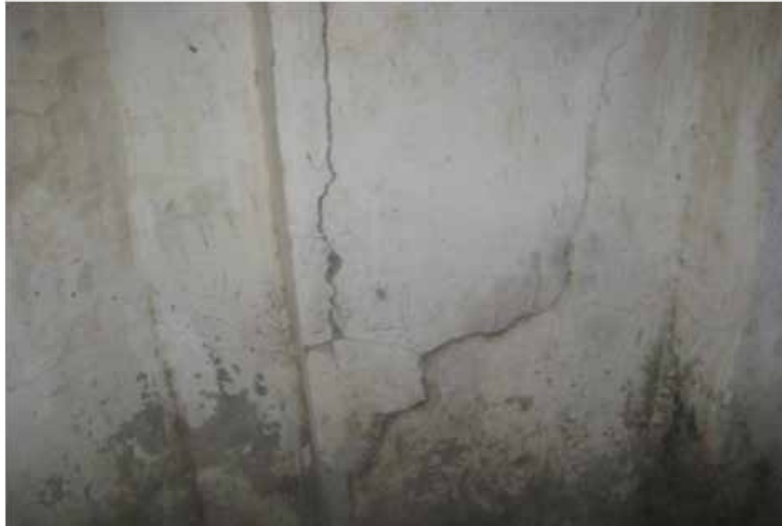
Image 6. Cracks at the intersection of walls
