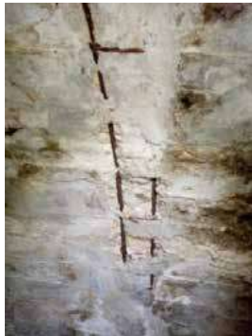
Figure 12. Underground culverts-arch's internal lining with strong steel corrosion problems and crystallized salts from concrete leaching (Mundo, 2019)
