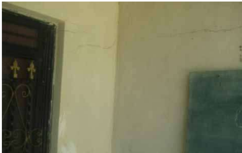
Image 5. Cracks at the intersection of walls
